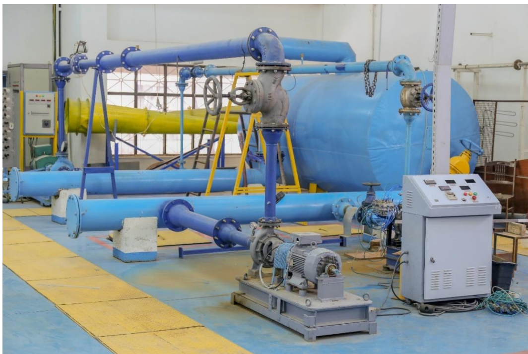
Fig. 14. Pumping system experimental setup.
